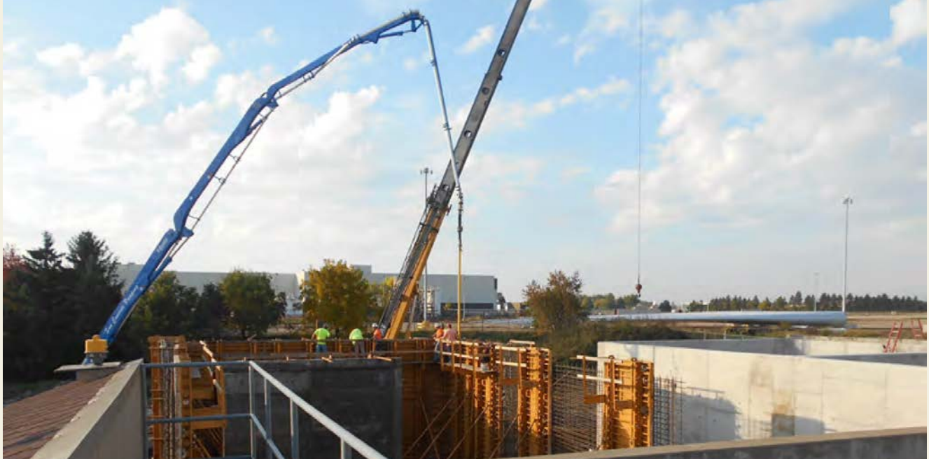
Using a cloud-based system has made Leander more productive on projects like the Eldridge Wastewater Treatment Plant.
